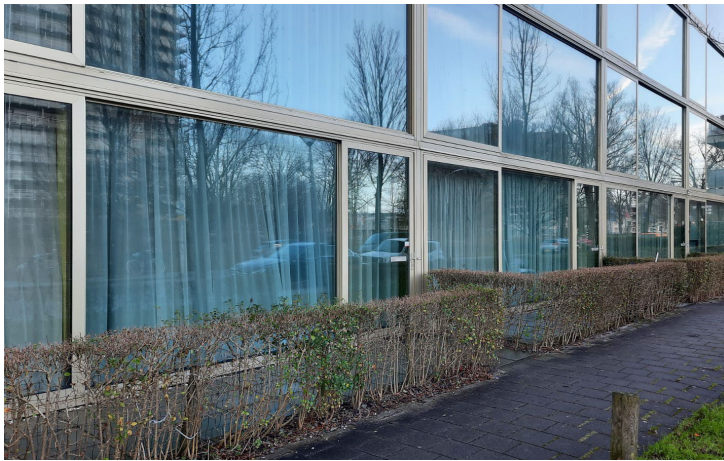
Figure 4.32 A facade in The Hague that is so transparent that paradoxically it is always closed
