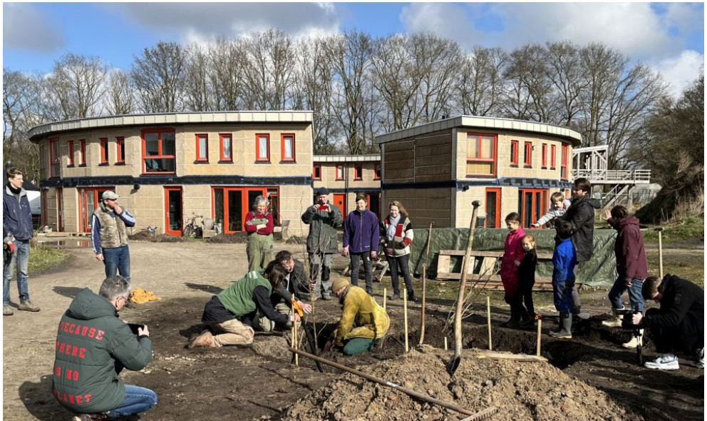
Figure 5.4 In 2022 Ecodorp Boekel became the first new build Dutch Vastgoedcoöperatie .
