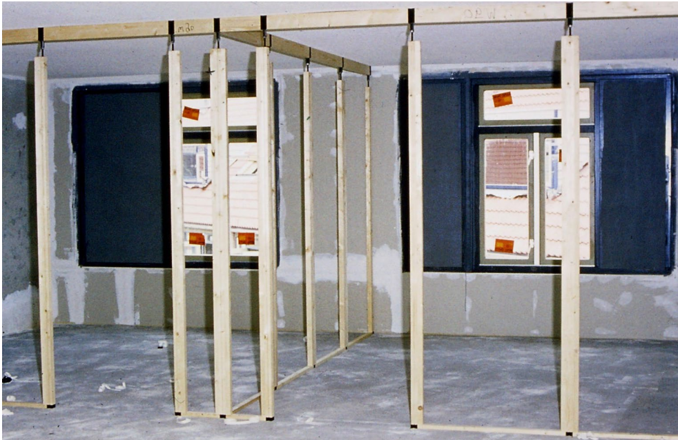
Figure 4.142 Flexible walls were at the core of the design of Gemeenschappelijk Wonen Nieuwegein by architect Flip Krabbendam. In 2010 a big renovation removed the flexible walls because of their bad sound insulation (Krabbendam, 2020).
