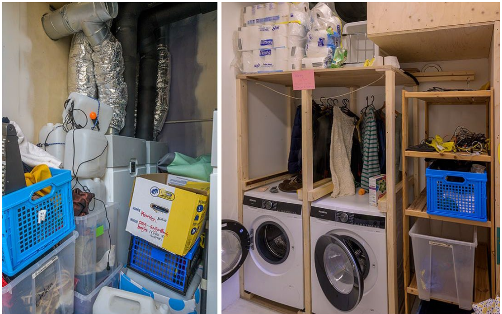
Figure 4.130 & 4.131 Some functional and necessary, but not so sexy, spaces in De Warren.
